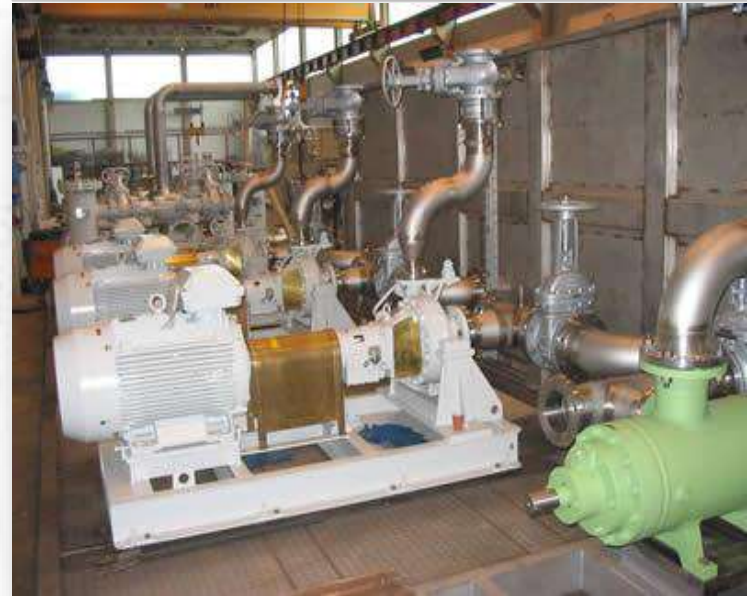
Pre-assembly & Testing Area
